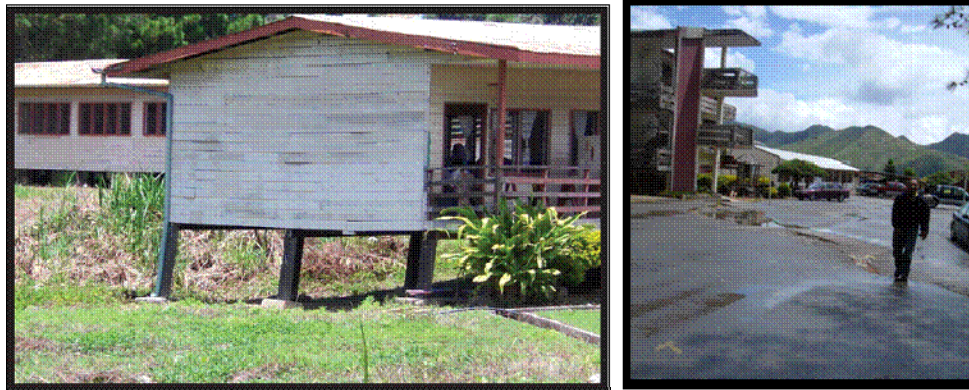
Figure 3: Infrastructures affected by active faults in Kundasang, Ranau
